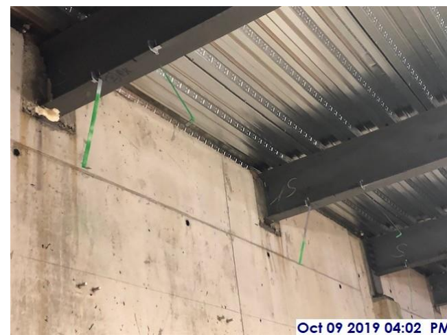
Hangars for HVAC, west sector basement
