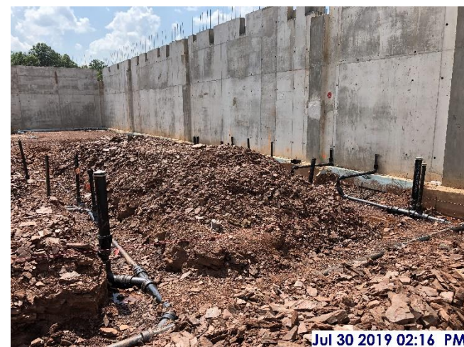
Underground plumbing, west sector
