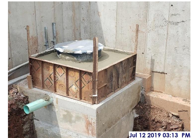
Ejector pit basin encased in concrete
