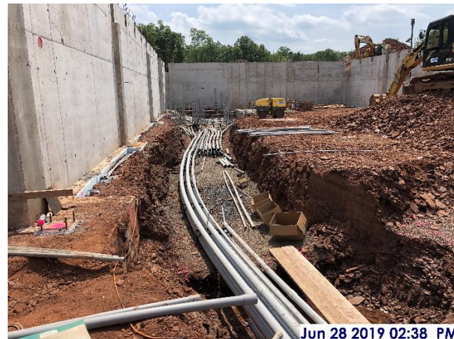
Underground electrical conduit, west sector
