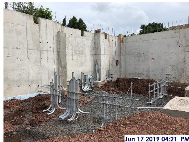
Conduit at Mechanical/Electrical Room, West Sector
