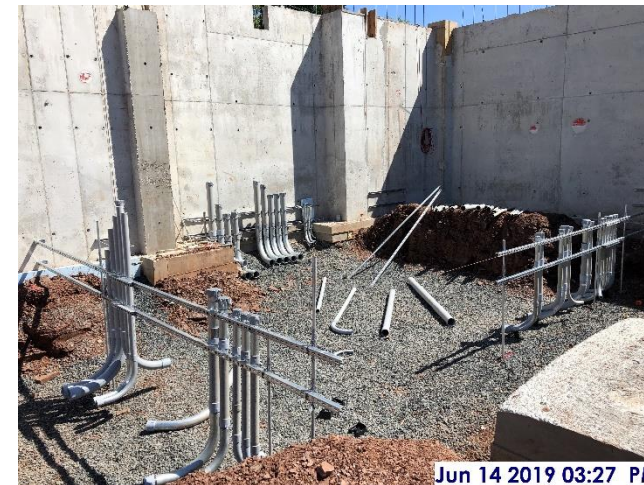
Unistrut & conduit in Mechanical/Electrical Room, west sector
