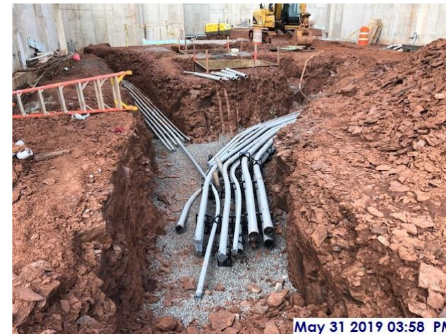
Underground electrical conduit in basement, center sector
