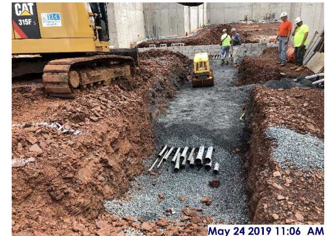
Basement electrical conduit, center sector
