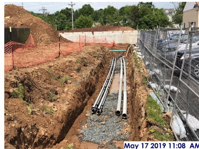
Underground conduit for primary electrical service
