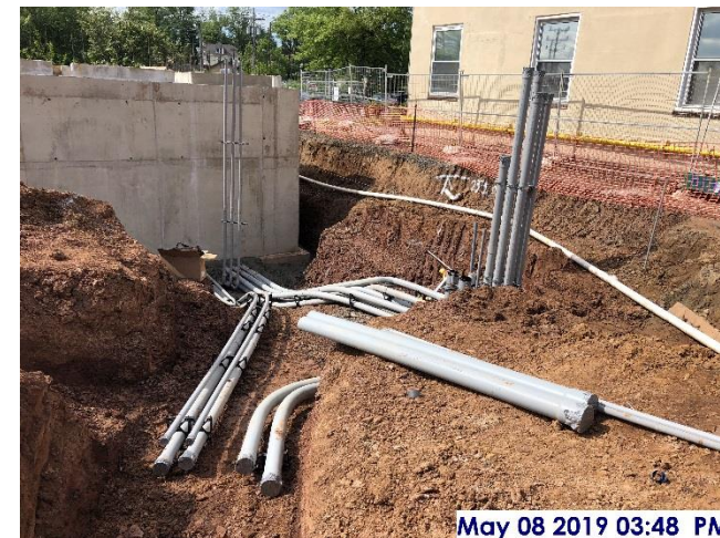
Underground conduit from main electrical room
