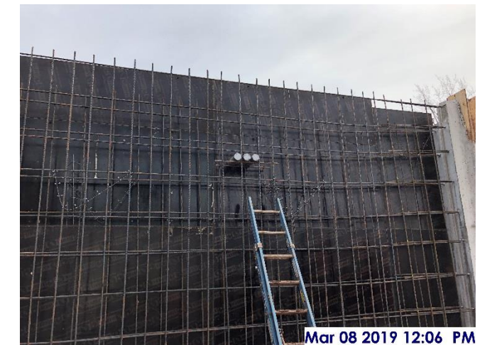
Penetrations and sleeves for electrical service
