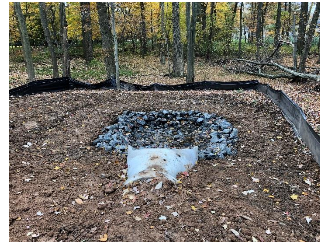
Rip rap stone at flared end of DPW storm line
