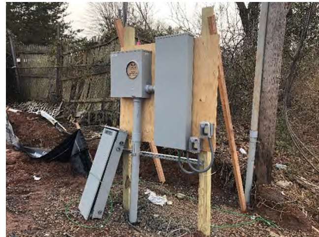
Temporary power for new Municipal Building
